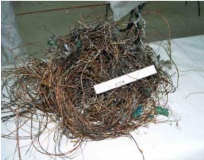
Figure 1: Bundle of heat-damaged wires
