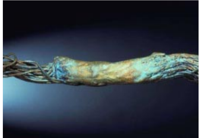
Figure 3: Left emergency DC bus cable
