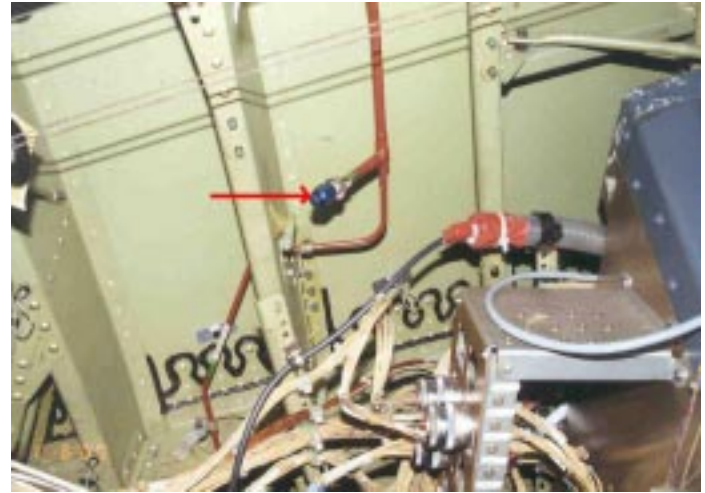
Figure 14: Crew oxygen line above cockpit ceiling showing an AN929-6 aluminum cap on the end of a stainless steel fitting
