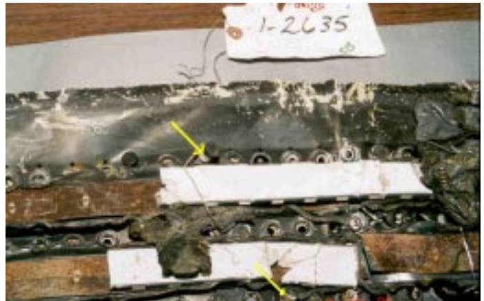
Figure 10: Upper right corner of overhead CB panel showing CB white trip indicator rings clean (upper arrow) and sooted (lower arrow)
